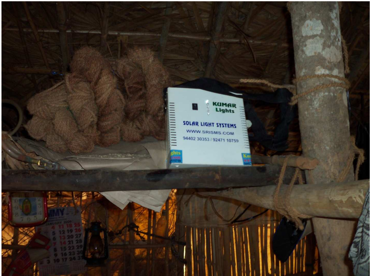
Solar light system on attic in a farmer home in Eluru
